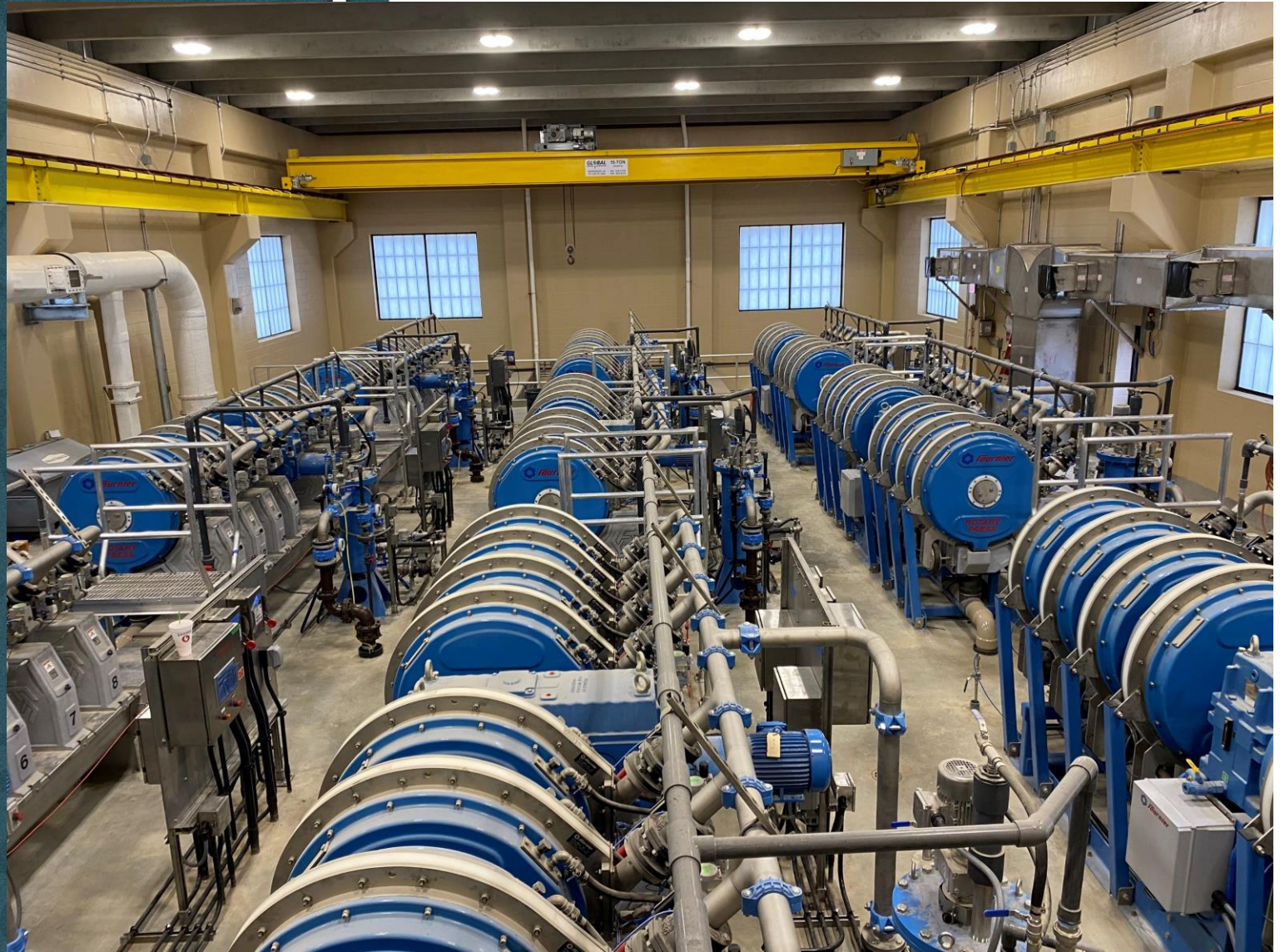
New Dewatering Equipment
