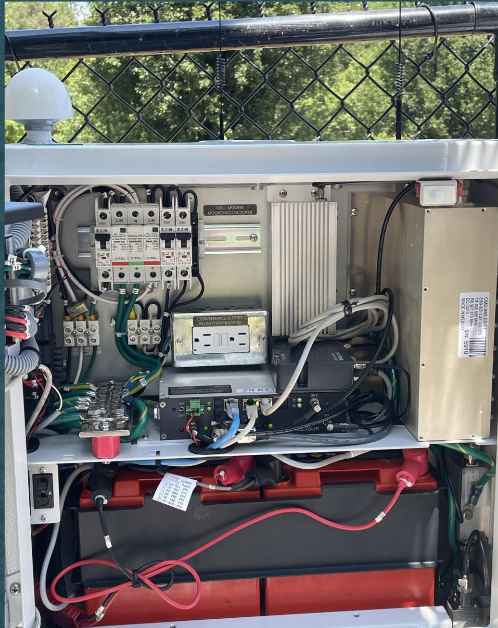
Sensus AMI Base Station Panel for Meter Reading
