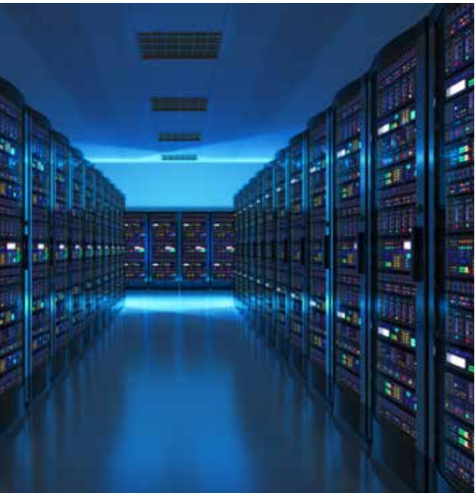
Data center server room (Source: Shutterstock)
