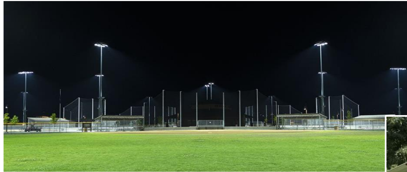
LED Field Lighting at Lanier Point
