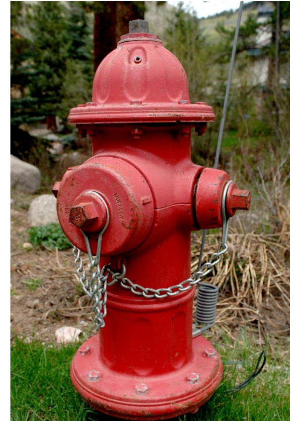
Public Fire Hydrant
