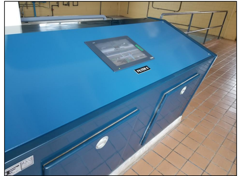
Riverside Filter Controls, 21 st Century
