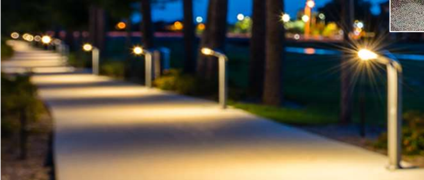
Rock Creek Greenway Lighting
