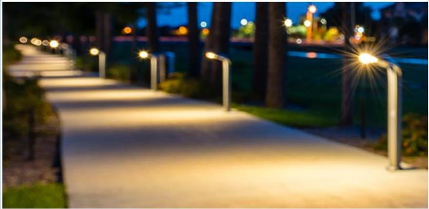
Greenway Lighting – RCG & MG
