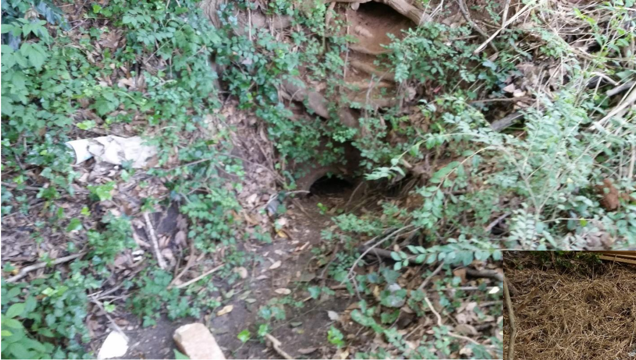
“Before”: Pipe is more than 50% obstructed.
